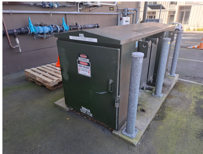
Figure 2. 300 kVA distribution substation at 222 Willis Street, Wellington
