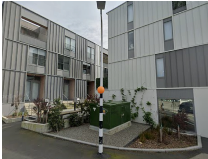
Figure 3. Urban distribution transformer installation in the Wellington CBD
