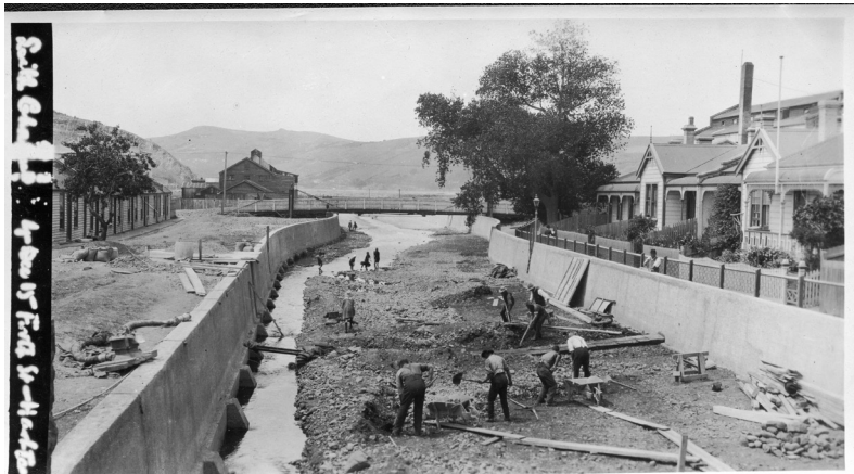
Figure 5: DCC Archives City Engineers Correspondence CE 2 3 39 1915. Laurel Bank is on the left in the image.
