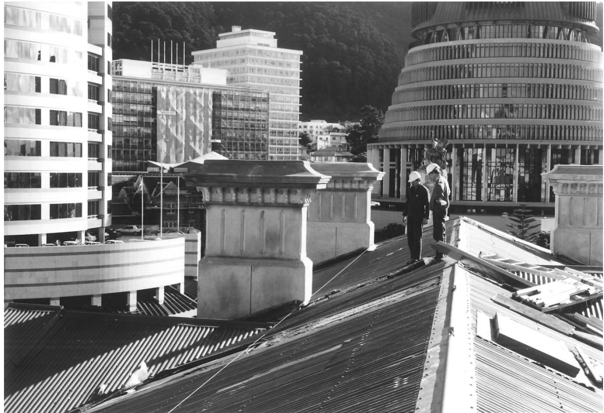
Figure 1: General view of chimneys on south wing roof during installation. Photograph 140795-165-22 "Conservation Record Form no. 145/2/2 Fireplaces/chimneys (20 October 1995)" File No. 13002-232 Ba Vol.1i, Heritage New Zealand Pouhere Taonga, Wellington.
